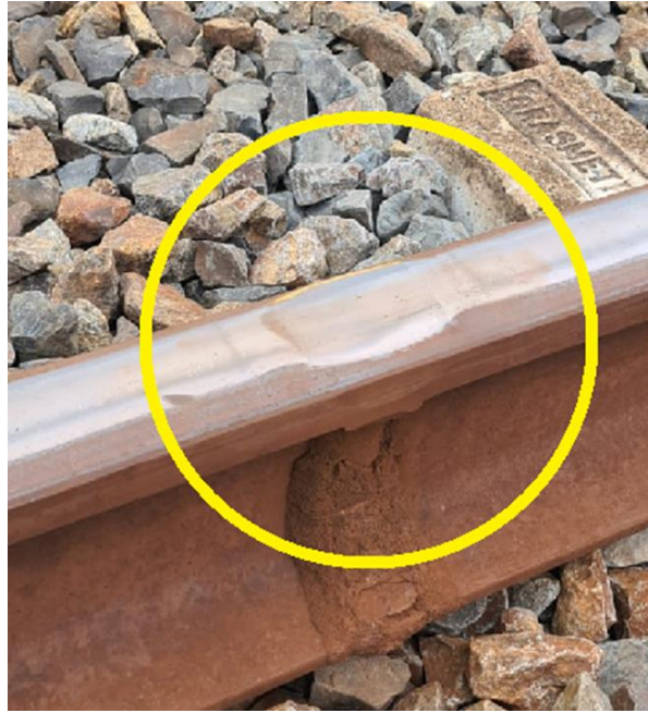
Image 5 - Welding problem in a section of the permanent way
