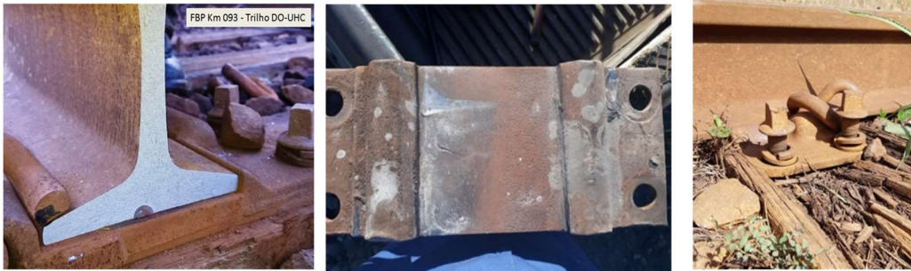
Figure 19: Examples of degraded support plate and impacts for rail and sleeper (Source: MRS Maintenance Report, 2023)
