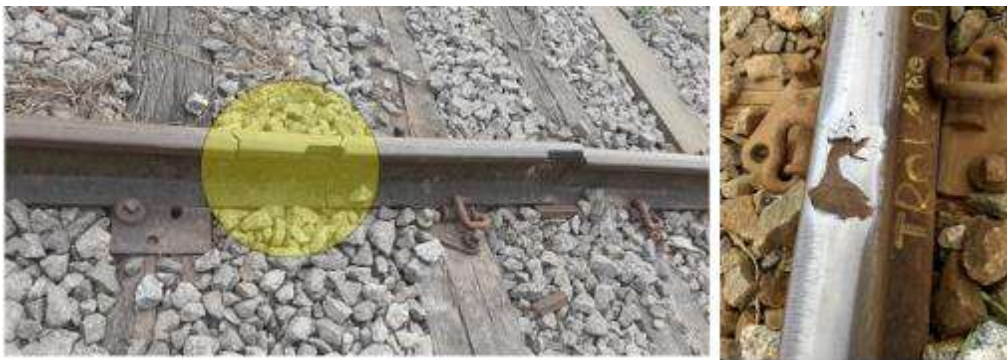
Figure 20: Examples of critical rail failures (Source: MRS Maintenance Report, 2023)
