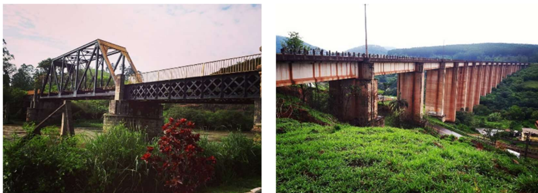
Figure 6: Riveted steel bridge from 1910s and prestressed concrete bridge from 1980s respectively (Source: MRS)
