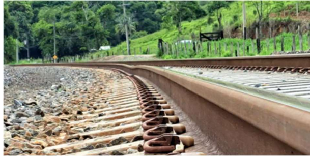
Figure 13: Deformation in the superstructure caused by low substructure support capacity (Source: MRS)
