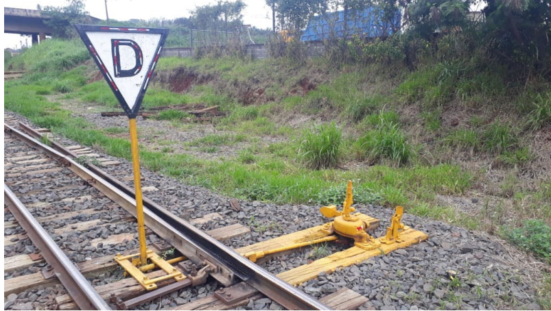
FIGURE 25 - DERAILER AND FLAG OF SWITCH ON DERAILMENT POSITION
