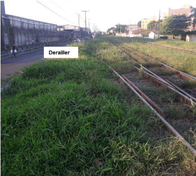
FIGURE 16 - EXCESS OF BUSH AT THE DERAILER REGION
