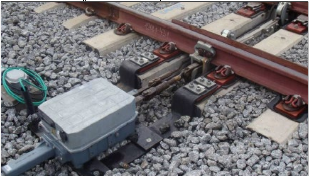
Figure 9 - Siemens S700K point machine mounted
