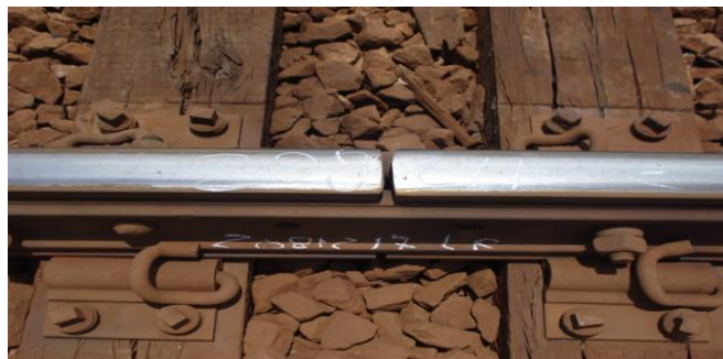
Figure 3 – Hanging/ in-balance rail Joint. Source: Authors
