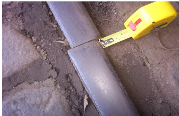
Figure 11 – Rail Misalignment at Gauge Line. Source: Authors
