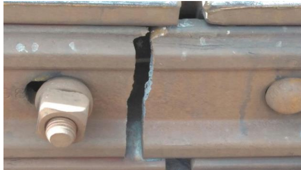
Figure 8 – Broken joint. Source: Authors
