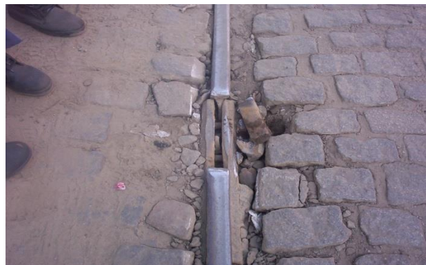
Figure 9 – Vertical Cracks on the Rail – (top rail crack). Source: Authors
