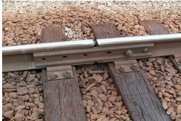
Figure 6 – Unconnected joint. Source: Authors
