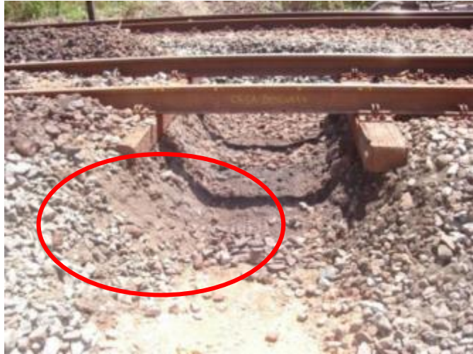
Figure 5 – Example of Ballast Contamination by
