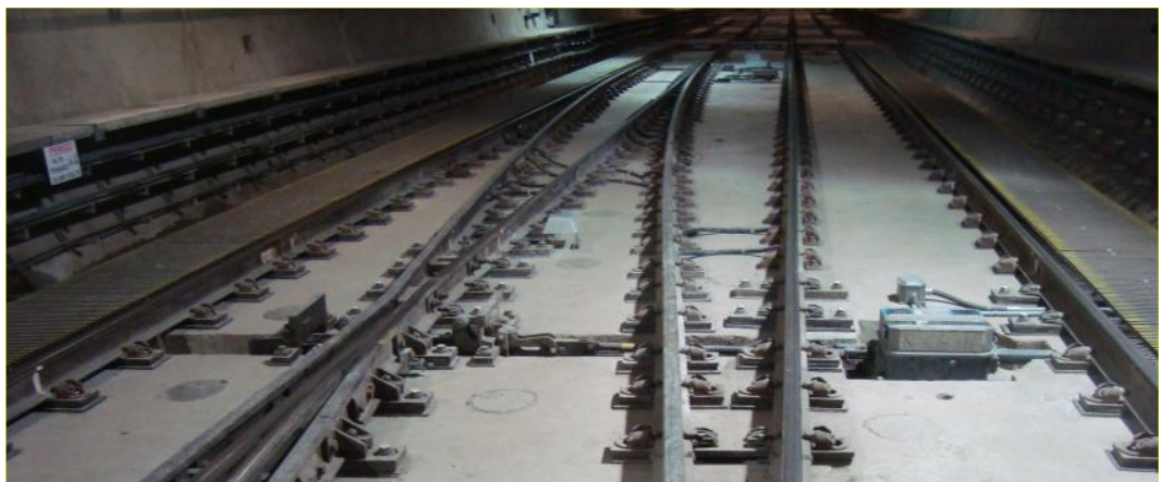
Fig 8: point machine for the switch rail (far) and for the moveable frog (near).
